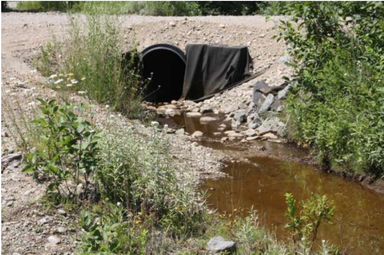
Figure 11: Creek Crossing in Tioweró:ton Experiencing Erosion Problems
